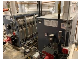
Boiler Room Alarms
