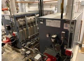
Boiler Room Alarms
