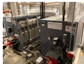
Boiler Room Alarms
