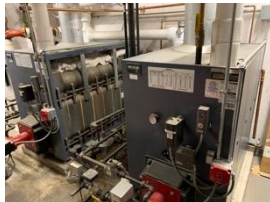
Boiler Room Alarms
