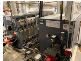
Boiler Room Alarms
