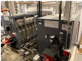
Boiler Room Alarms
