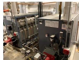
Boiler Room Alarms
